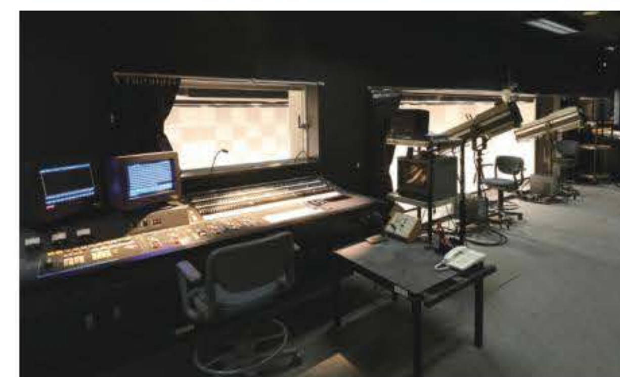
音響・照明設備 Acoustic and Lighting facilities
